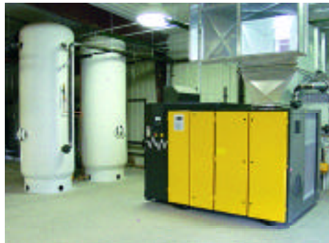
A 180-hp screw compressor with variable-frequency control.
